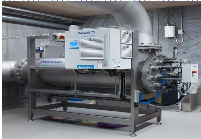
Ultraviolet water disinfection system
