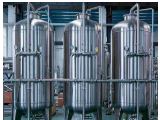
Pic.1 Water filter system
